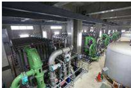
Ceramic membrane filtration system (Delivered to projects including Kawai Water Purification Plants in Yokohama)
