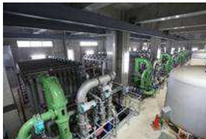
Ceramic membrane filtration system (Delivered to projects including Kawai Water Purification Plants in Yokohama)
