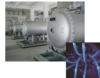
Ozone processing system
