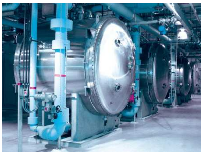
◀ Ozone processing system (Delivered to Boston, the US, and others)
