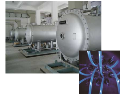
Ozone processing system
